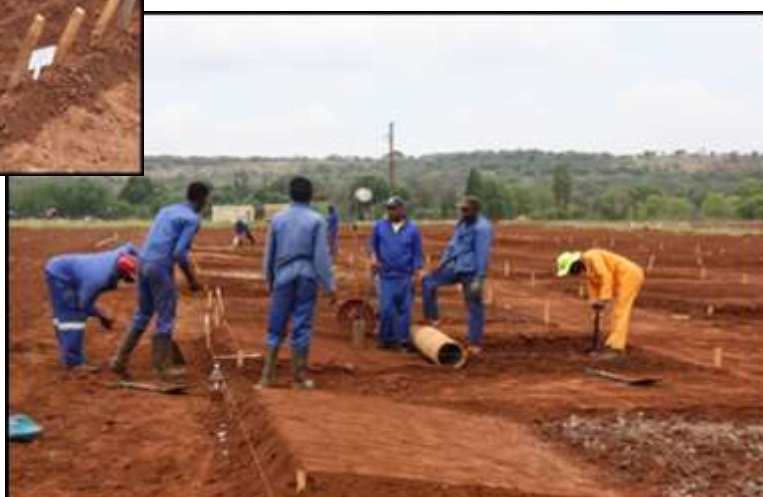
Figure 7. Compaction of the runoff collection areas of the in-field rainwater harvesting and conservation technique at Roodeplaat, ARC-VIMP.
