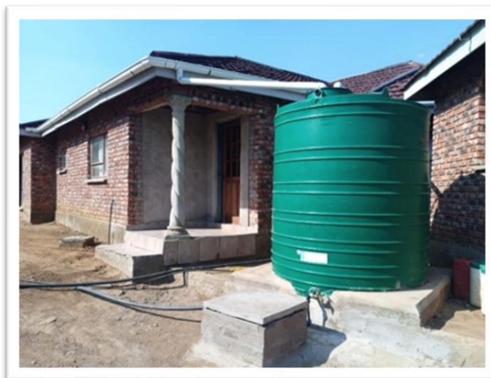
Rainwater harvesting tank with booster pump
