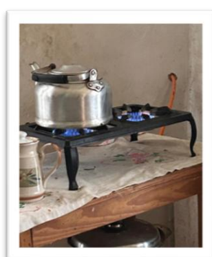
Operational gas stove – status at 18 months post-installation, indicating well fed biogas digester with good pressure
