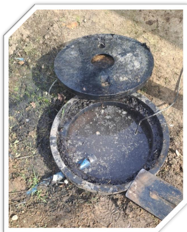
A manhole at one of the study participants' wastewater treatment facilities
