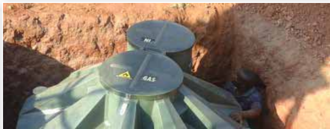
6m 3 pre-fabricated biogas digester.
