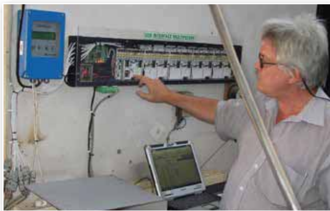
Sprinkler testbench control system to determine the performance of sprinklers.
