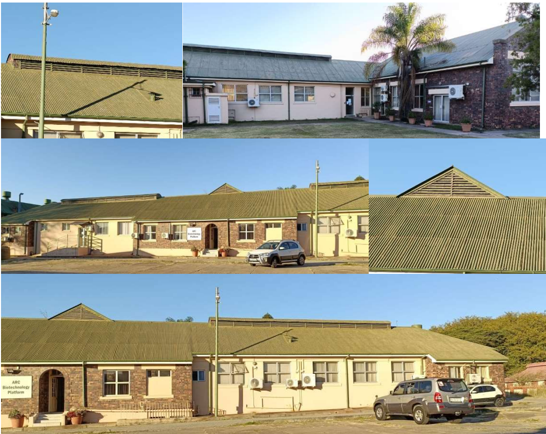
Figure 1. Biotechnology Platform building's roof, wooden louvres, gutters, downpipes and Fasi boards showing that will require cool surface prep and painting.
