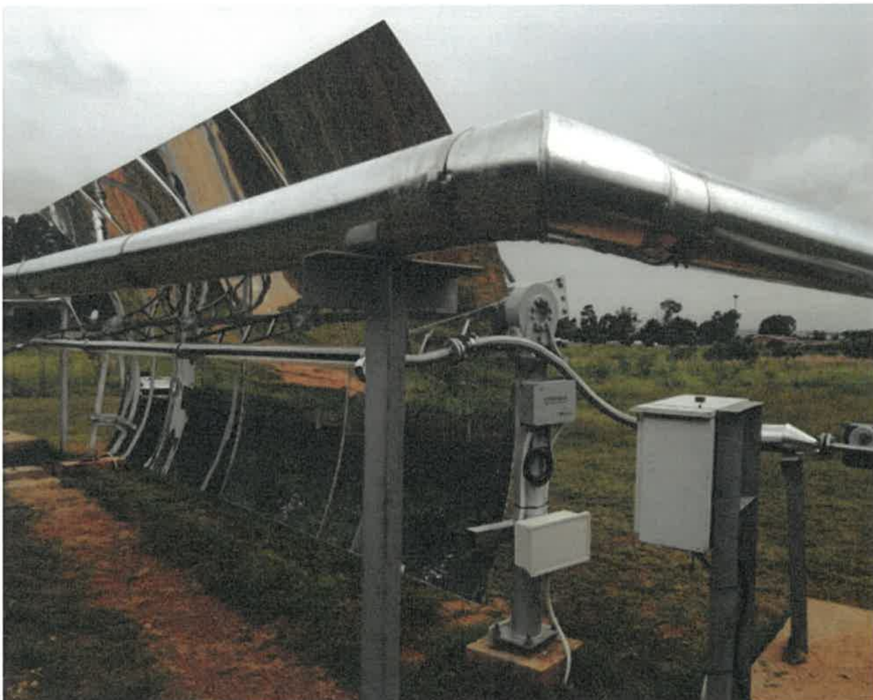
Figure 1: Parabolic Trough System, ARC-AE, Silverton Campus
